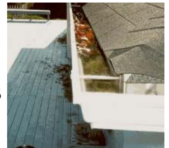
Clogged rain gutters
